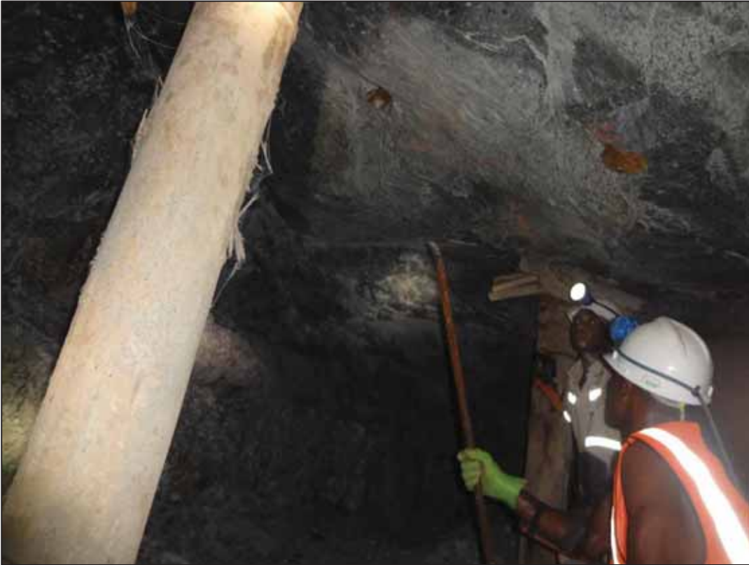
Figure 60: Absence of gasket/ hand guard due to it easily sliding off the bar (Mining House D)
