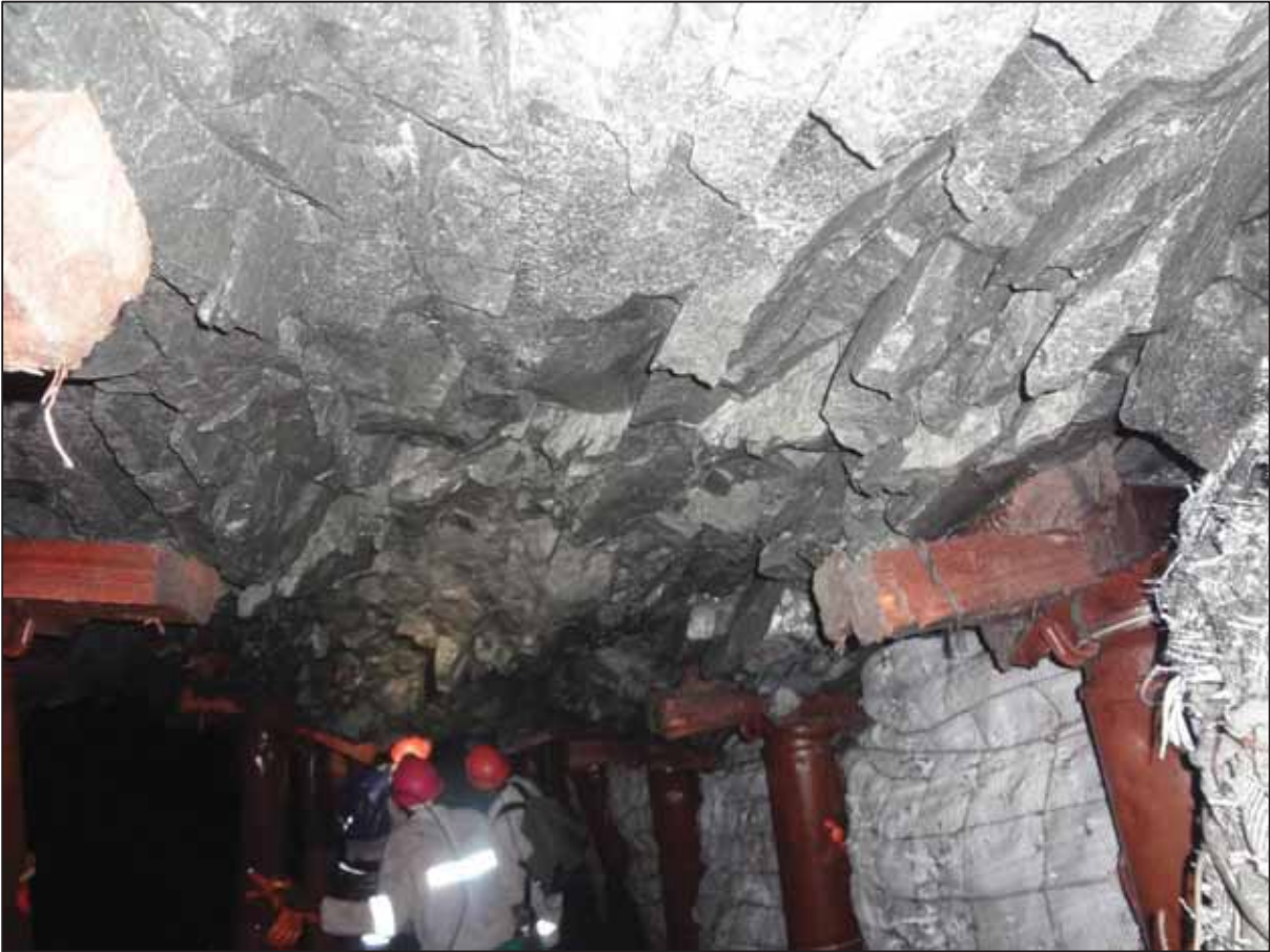
Figure 64: Steeply dipping joints in hanging wall lava (Mining House E)
