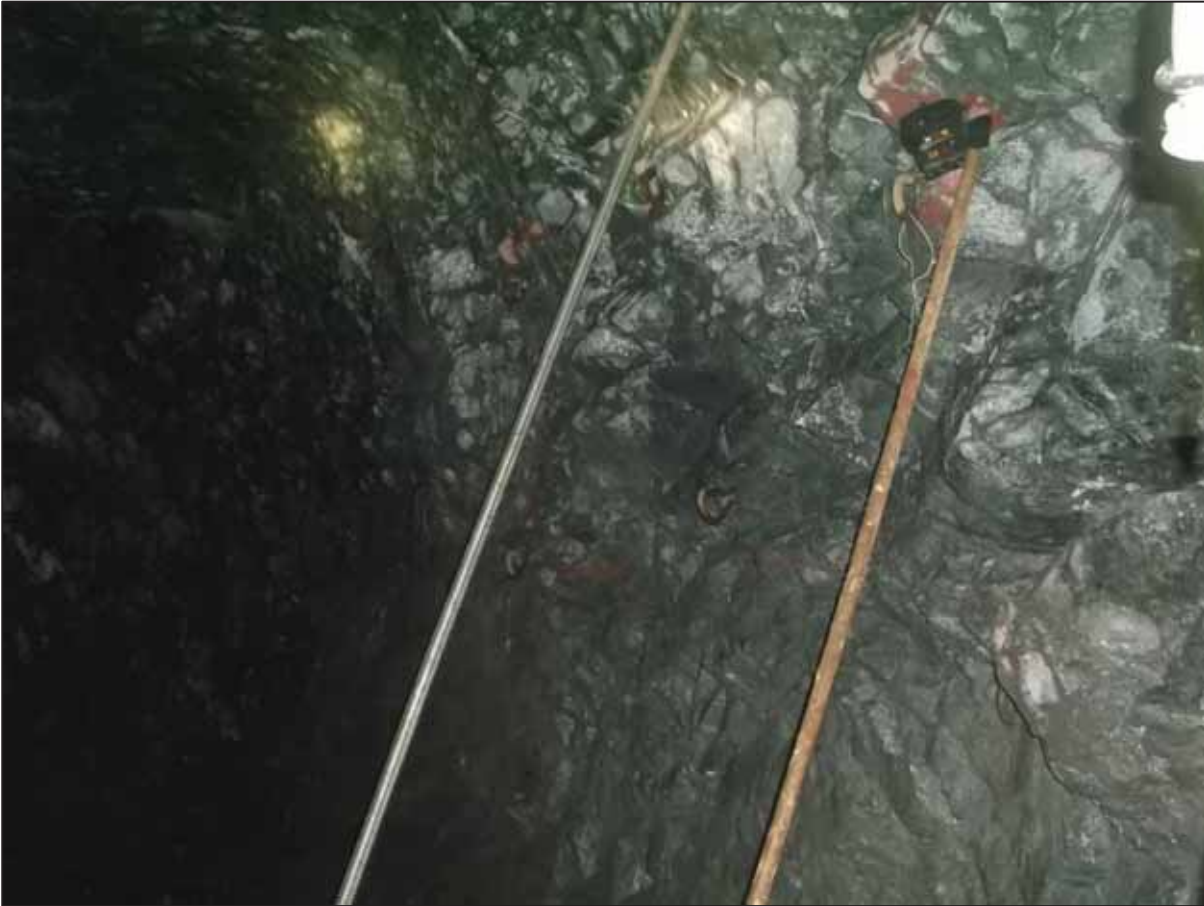
Figure 62: Pinch bar ready to be used for barring with no gasket fitted on (Mine 7)
