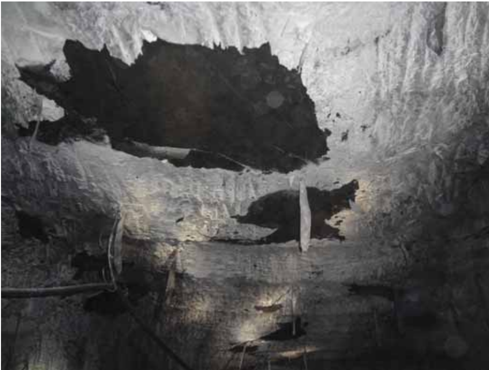
Figure 43: Typical slabbing and fall outs in a dyke area of Top Seam (Mine/ Shaft 3)
