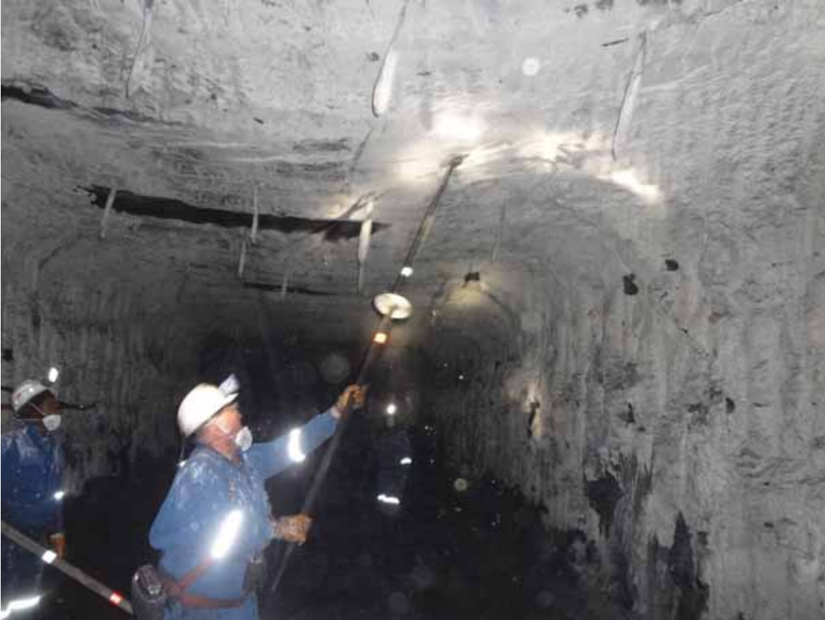
Figure 39: Barring with a conventional hollow steel tube pinch bar with the secured steel gasket (Mining House F)
