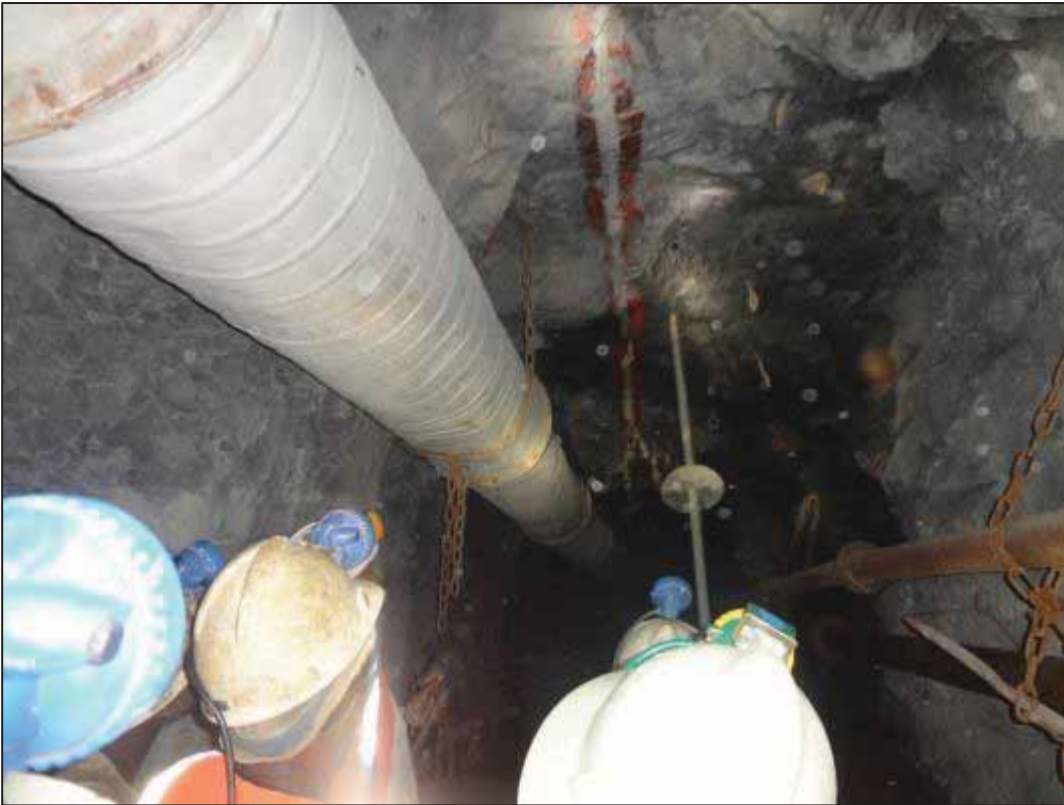
Figure 76: Development excavation greater than 2m high in a gold mine with poor hanging wall conditions and overhanging side wall (Mining House D)
