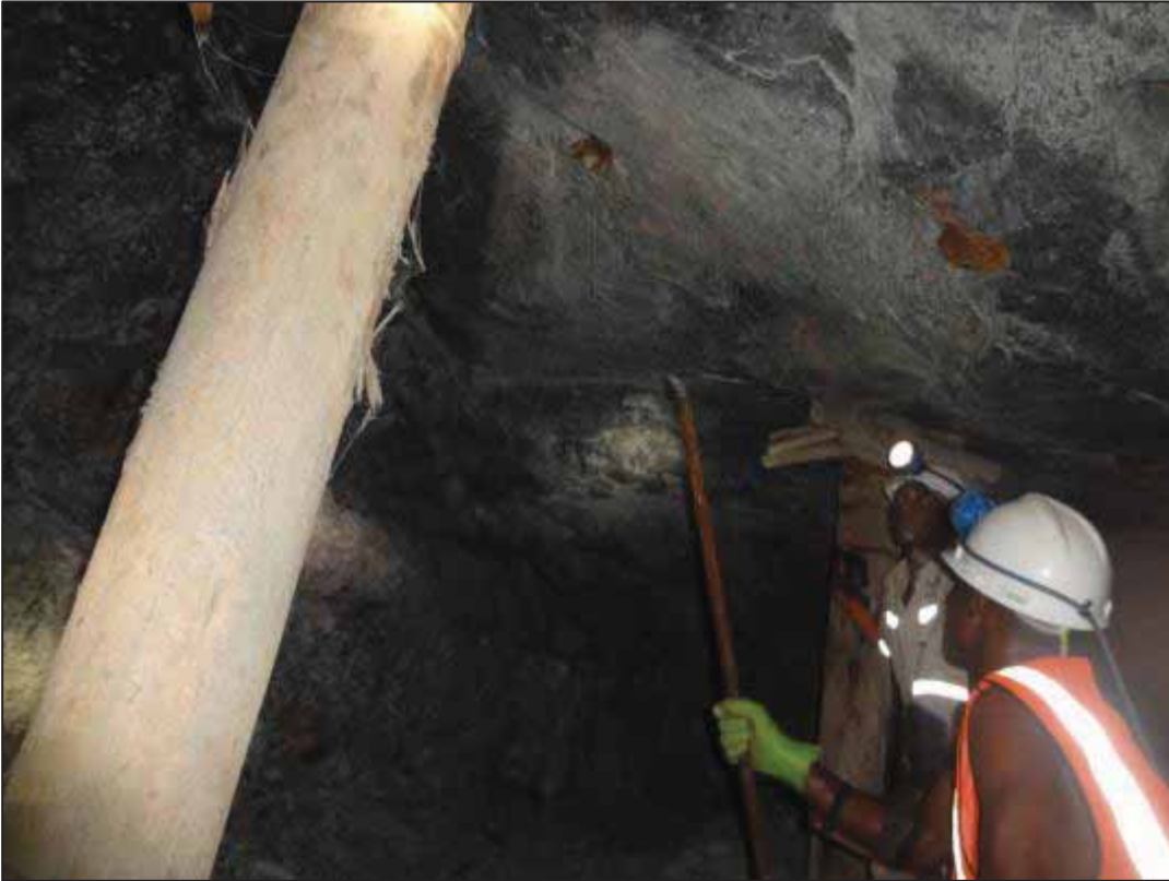
Figure 68: Poor barring practice with the absence of gaskets/ hand guards due to it easily sliding off the bar (Mining House D)
