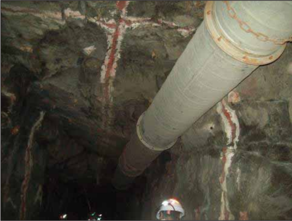
Figure 43: Development excavation greater than 2m high in a platinum mine with poor hanging wall conditions and overhanging side wall (Mine 9)
