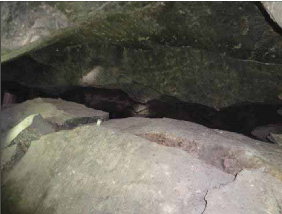
Figure 39: Fall-out due to dome feature and associated low angle joints (Mining House C)
