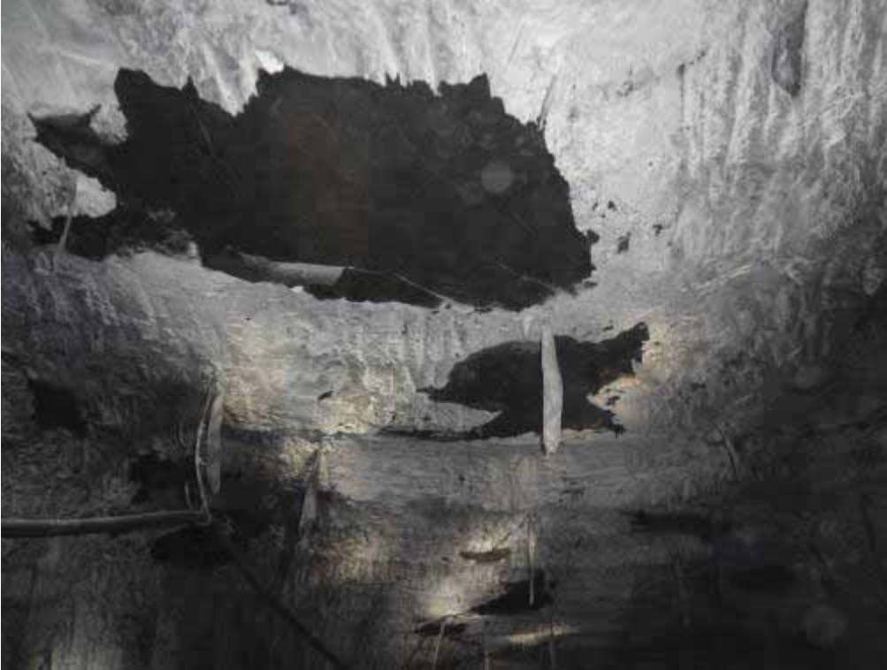
Figure 54: Typical slabbing and fall outs in a dyke area of Top Seam (Mine/ Shaft 3)
