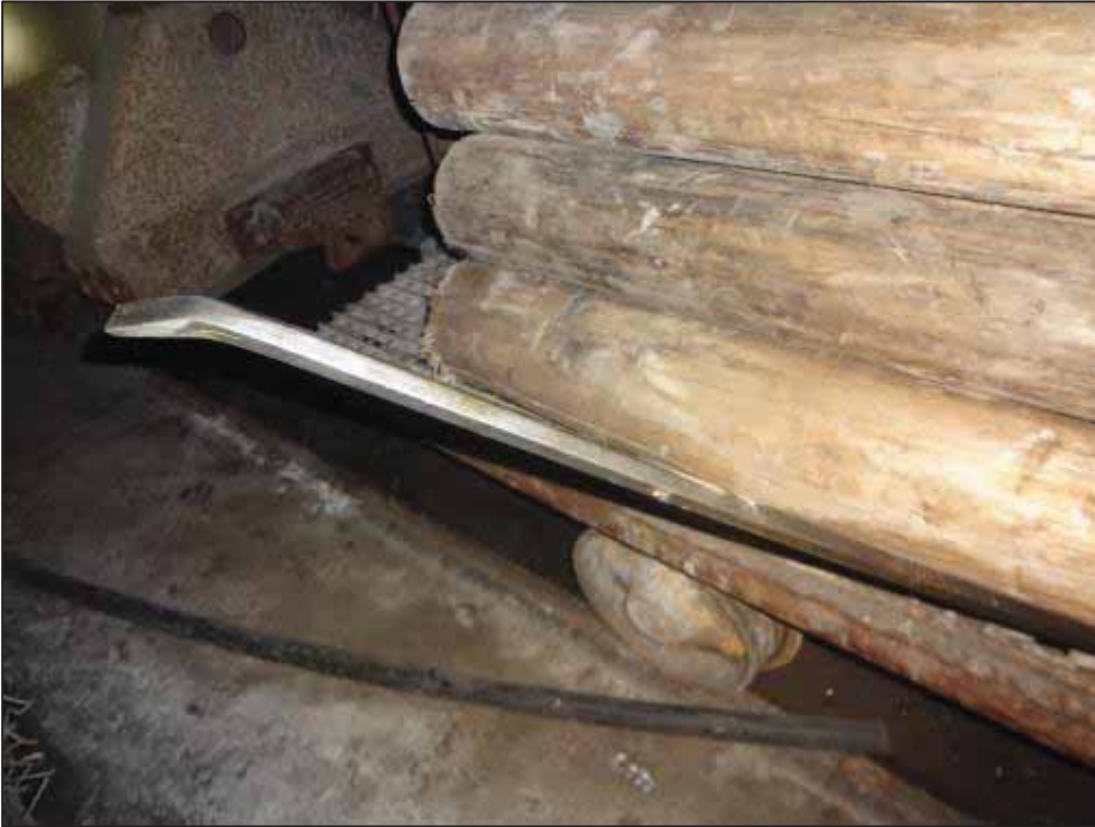
Figure 37: Incorrect usage of pinch bar to hold mine poles in place on 'skip' - this is a task not intended for the equipment and the sharp point poses a hazard to personnel travelling alongside the tracks (Mine 11)
