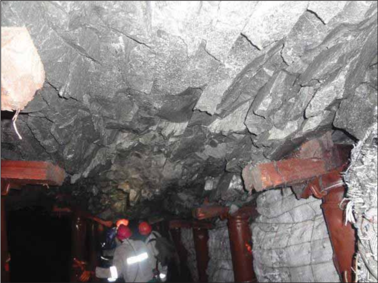
Figure 72: Steeply dipping stress-induced fractures in hanging wall lava (Mining House E)
