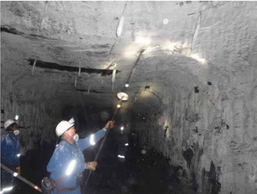
Figure 51: Barring with a conventional hollow steel tube pinch bar with the secured steel gasket (Mining House F)
