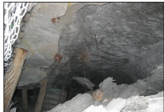
Figure 3: Dense fracturing of exposed Norite leading to collapse.
