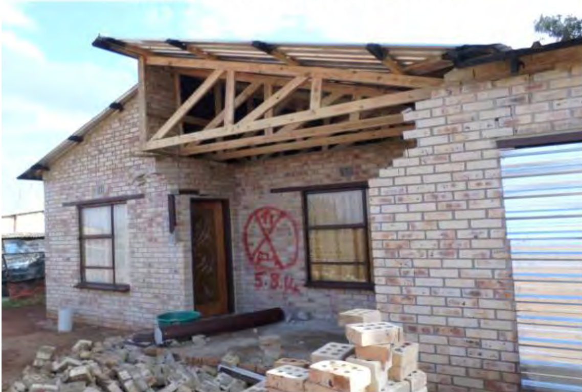
Failure of cantilever wall
