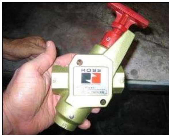
Figure 4: Isolation point for equipment with air starts
