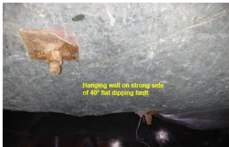
Photo taken of hanging wall & support immediately down-dip of the 40° flat dipping fault – TARP 2 conditions
