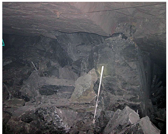
Top view from 13 West RSE 14 (Damp mud infill on hanging wall)
