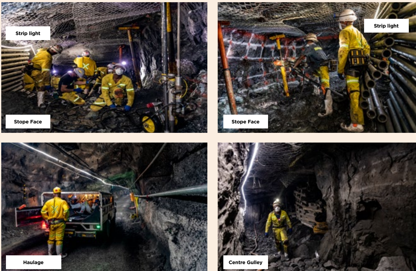
Figure 6: Strip lights installed on reef at Eland mine
