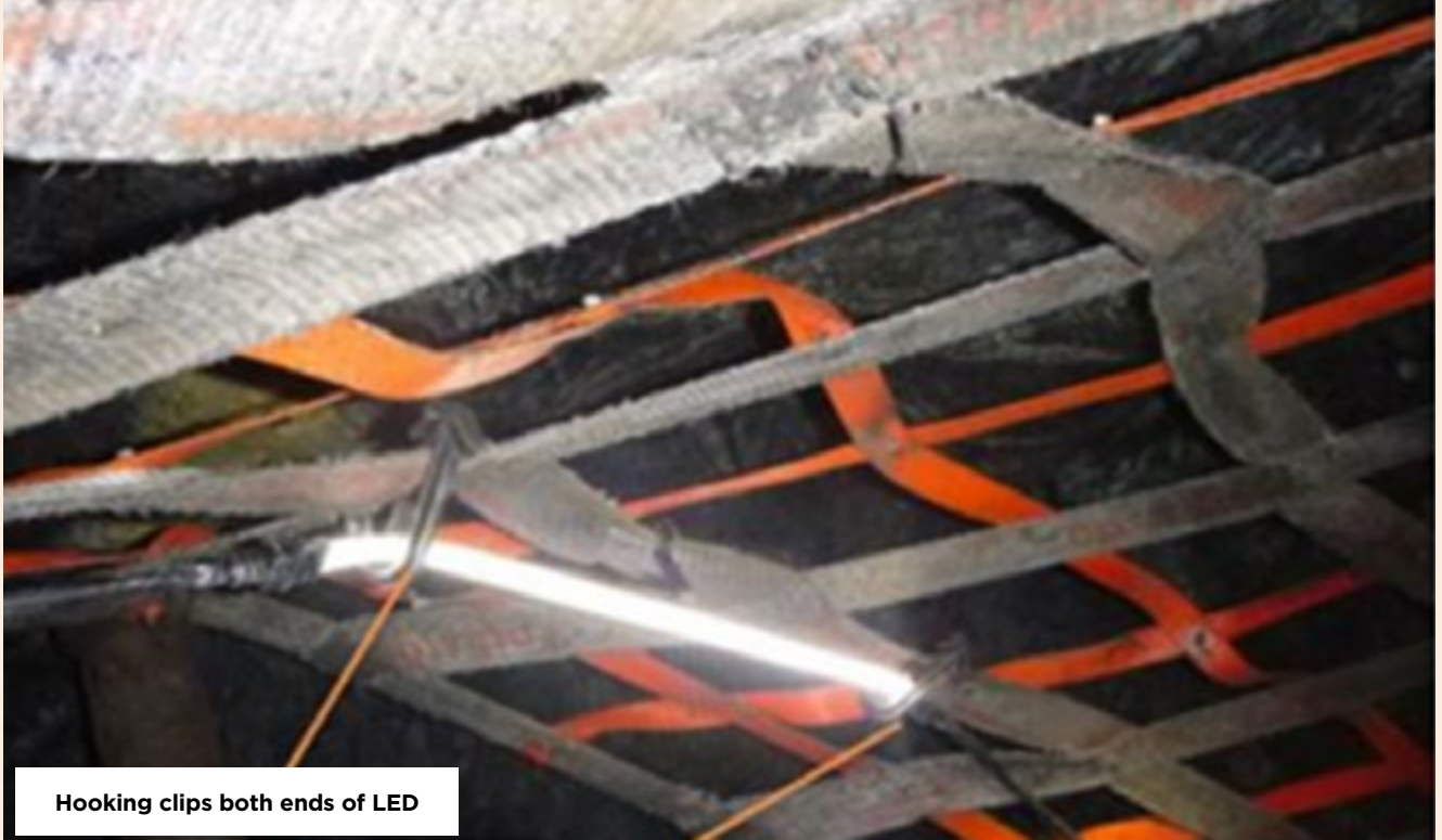
Figure 7: LED strip lights attached to safety net at Dishaba
