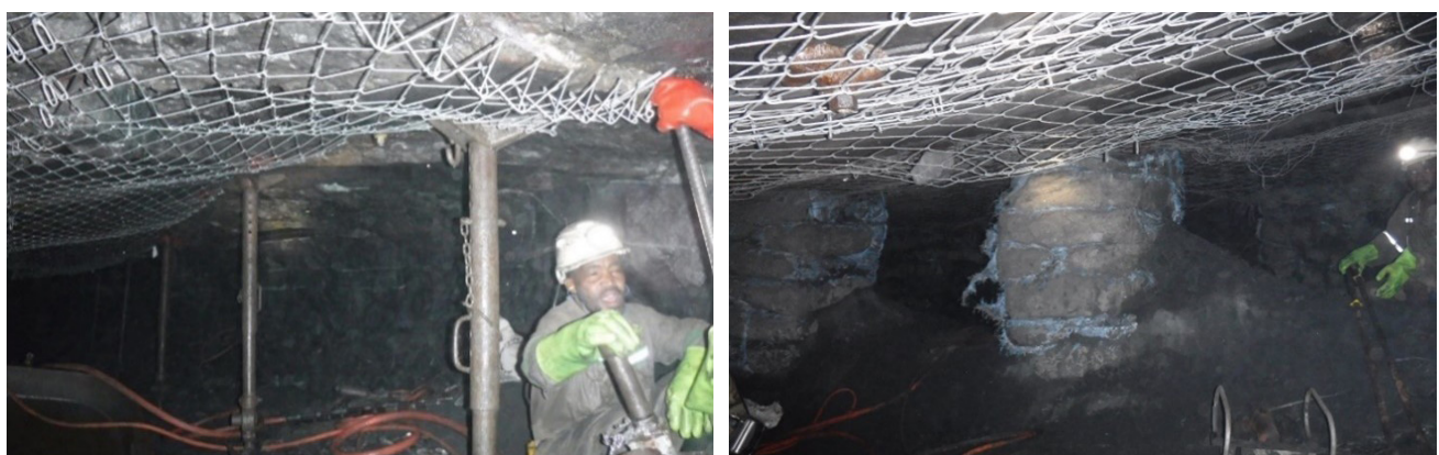
Figure 17: Permanent workforce areal mesh installation at Saffy Shaft while negotiating TARP 3 conditions
