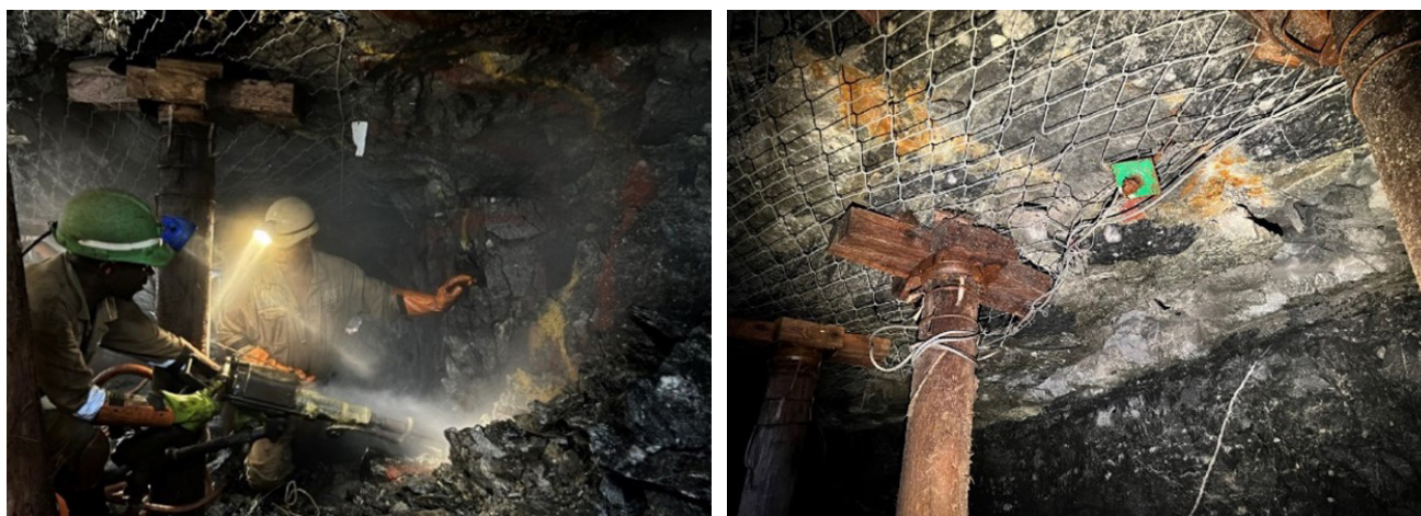
Figure 16: Permanent workface areal mesh installation at Mponeng Mine with elongate support installed close to the face
