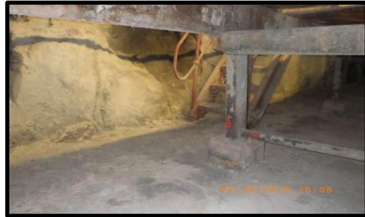
12 Level Belt section – dust & ore accumulation removed under and around the belts
