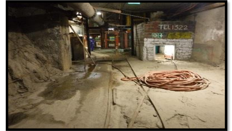
28 Level towards the fridge plant – dusty station areas
