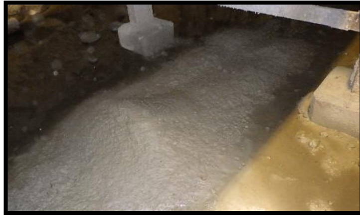
12 Level Belt section – dust & ore accumulation under and around the belts
