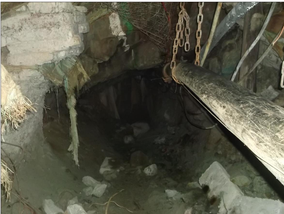
Figure 91: Poor housekeeping in gully area
