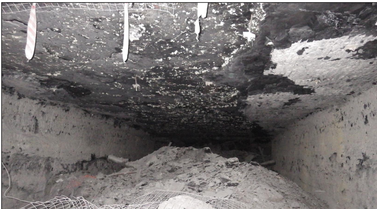
Figure 58: Scaling into roof by operator - Top RHS of picture
