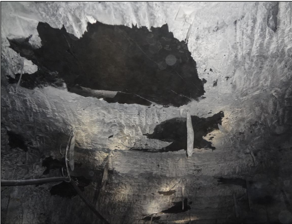
Figure 39: Poor Roof conditions
