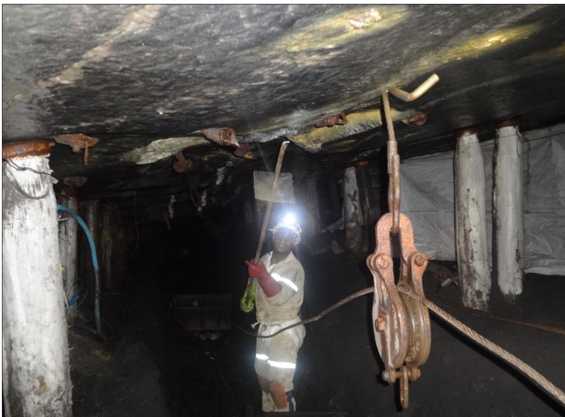
Figure 21: Barring in strike gully
