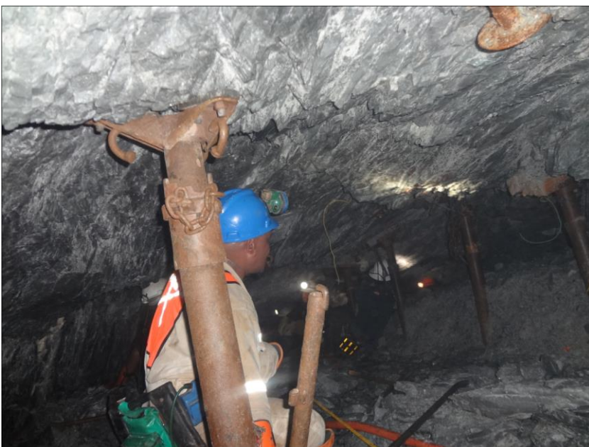
Figure 26: Poor HW condition
