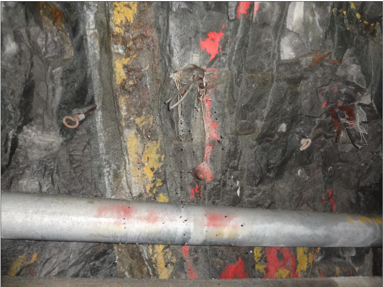
Figure 10: Fault demarcation - Note the fissure flow through anchor - not grouted well
