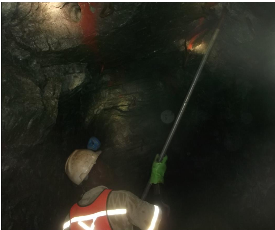
Figure 89: Barring in stope. No gasket on pinch bar
