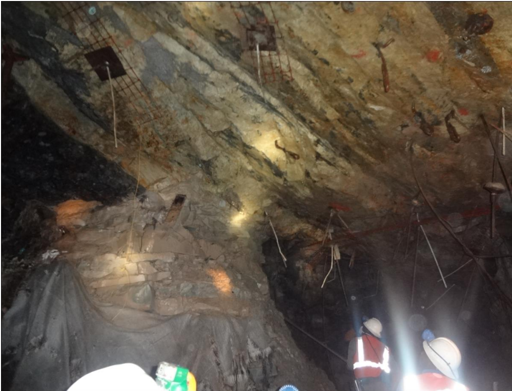
Figure 33: Exposed Backfill bags and poor HW condition
