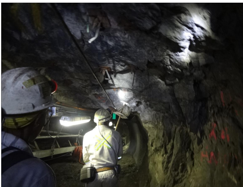
Figure 14: Barring at conveyor belt area
