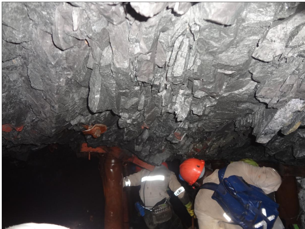
Figure 36: Steeply dipping joints and stress induced fracturing in the HW
