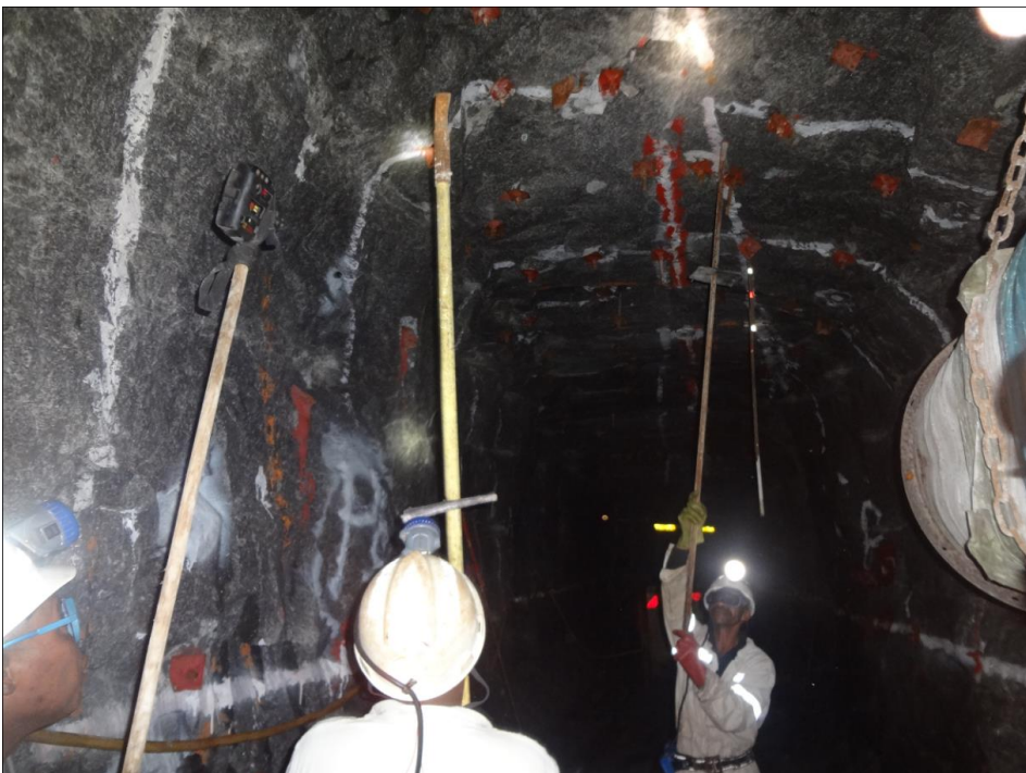
Figure 22: Incorrect positioning directly under the rock being barred, and note the position of the gasket
