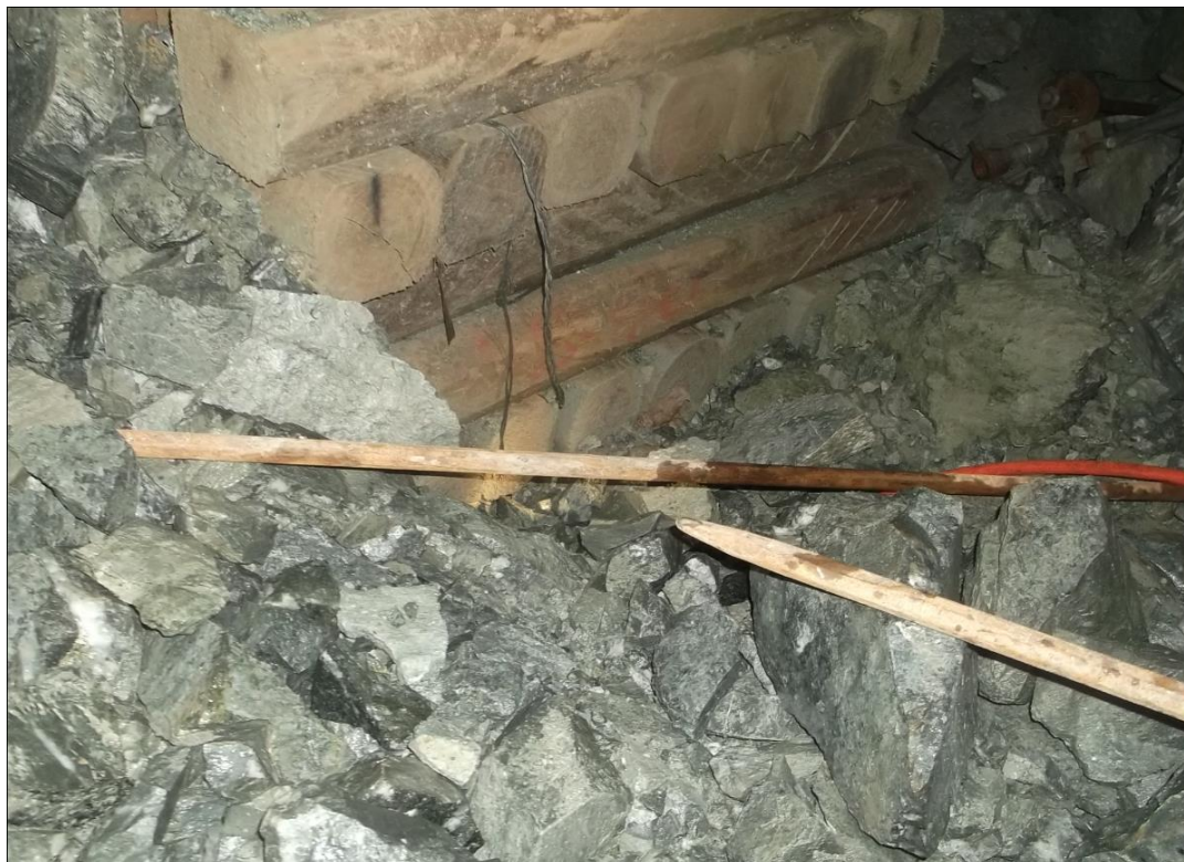
Figure 93: Old, rusted and blunt pinch bars without gaskets
