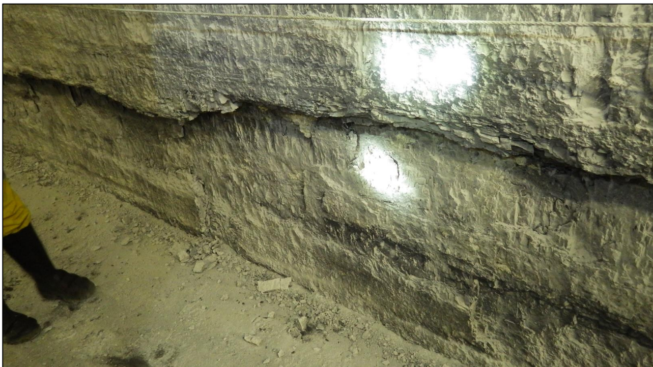
Figure 57: Scaling in rib sides
