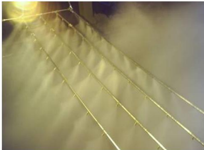
Figure 18: Nozzles emitting fine water sprays. (South Deep Mine; source Envidroclear)
