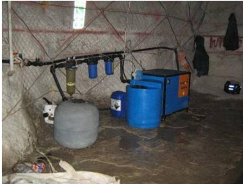
Figure 24: Fogger dust suppression system pump, motor and mixing pump. (Source Envidroclear)
