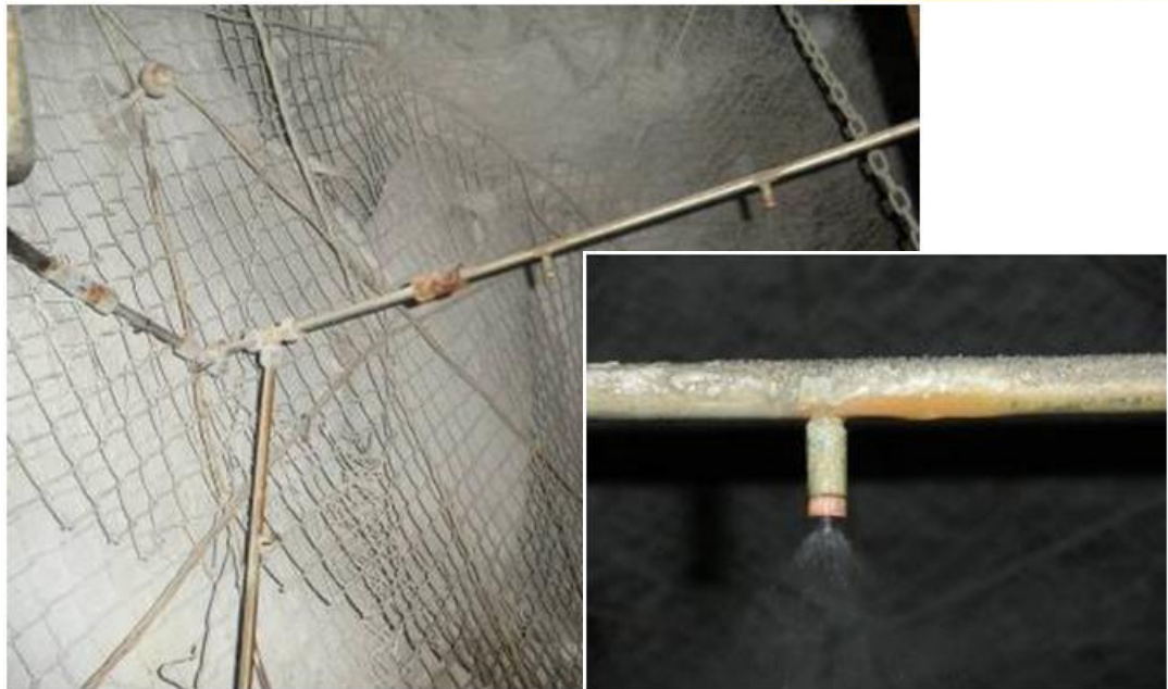
Figure 17: A section of a vapour curtain with a close up of a nozzle. (Great Nologwa Mine; source Envidroclear)
